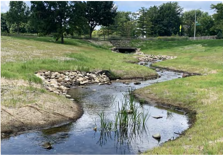
MEANDER CHANNEL SECTION WITH EXTENDED STONE TOE PROTECTION & BENCH (APEX OF MEANDER) NO SCALE
