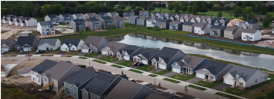
During the past fiscal year, significant progress has been made on the Trails of Woods Creek, a 279-unit residential development featuring homes ranging from $294,000 to the upper $400,000s.
