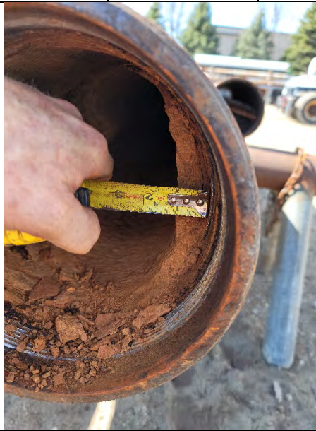
Over 1" of mineral buildup in ID of Column Pipe
