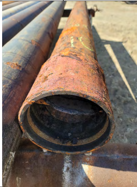
8" surge control valve, flappers are erosion
