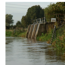
Raw Water Collection and Intake
