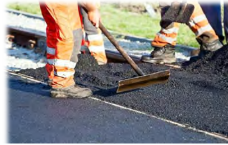
The MFT Fund assigns resources for repairing and resurfacing Village streets for improved travel
