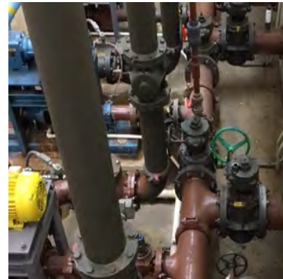
Primary Sludge Pumping Improvements brings automation to solids handling at the WWTF.
