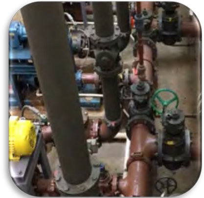
Primary Sludge Pumping Improvements brings automation to solids handling at the WWTF.
