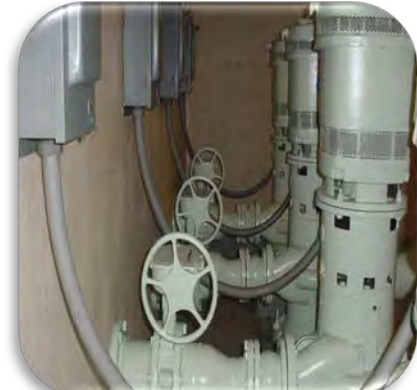
High Service Pumps at Water Treatment No. 2 to receive premium efficient motors and VFD's.
