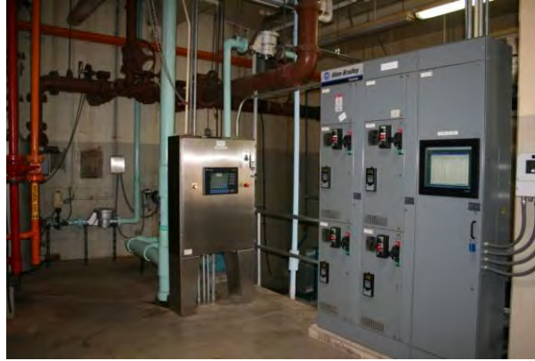
SCADA system at Wastewater Treatment Facility
