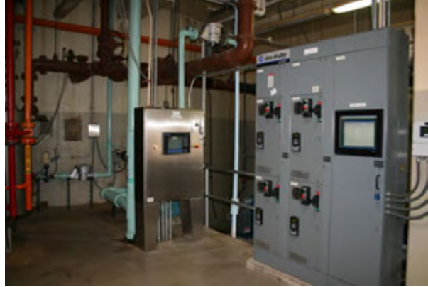
SCADA system at Wastewater Treatment Facility
