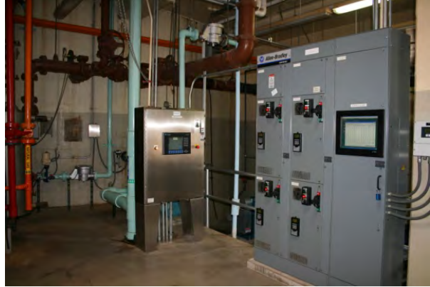
SCADA system at Wastewater Treatment Facility
