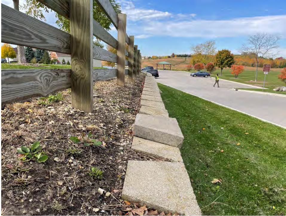
Top of Wall Looking West – Wall is Leaning Forward - Note that the Standard Batter for an Anchor Diamond Wall is 10.6^\circ Back. Front Face Angle Measured Up to Approximately 89^\circ (Up to 10^\circ Forward)
