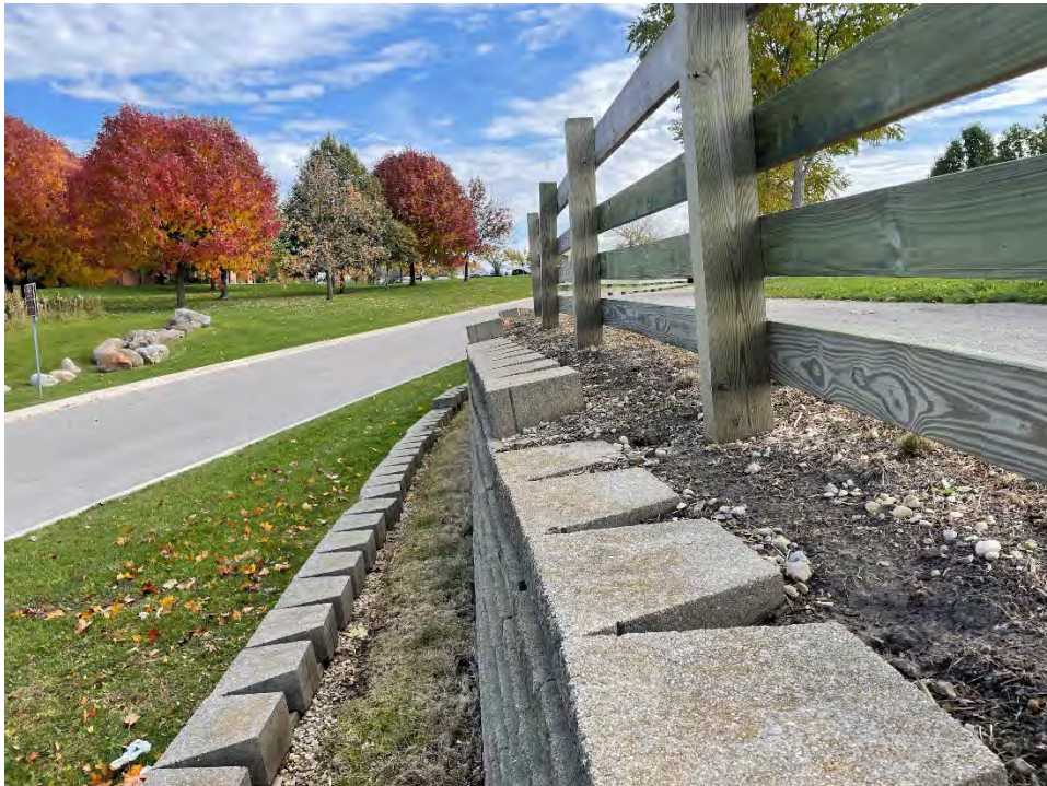
Upper Tier Looking East – Wall is Leaning Forward
