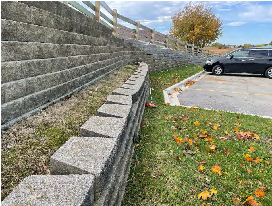
Lower Tier Looking West – Wall is Leaning Forward
