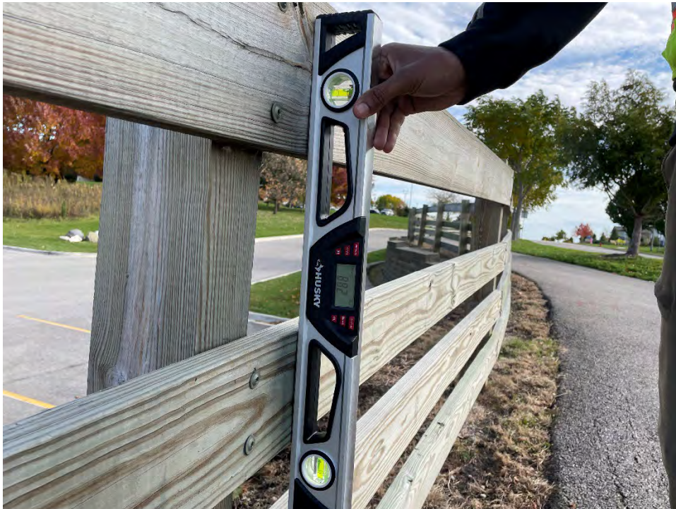
Wooden Railing Leaning – 88.2° at 60' from West End of Wall, 84.1° at 80' from West End of Wall (Railing is Leaning Towards Wall)
