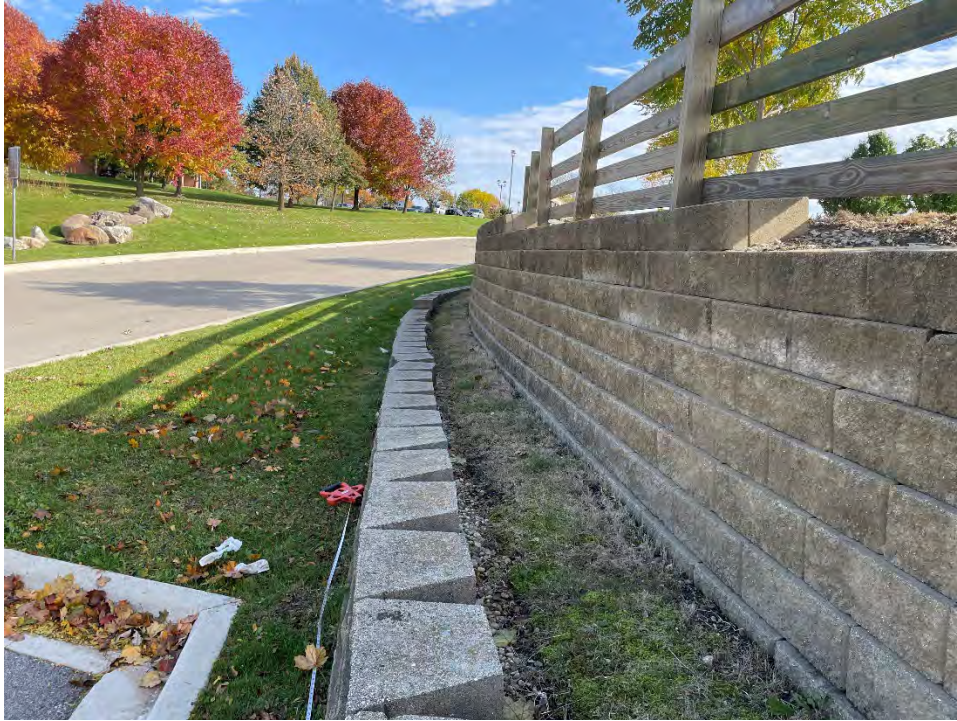
Lower Tier Looking East – Wall is Leaning Forward
