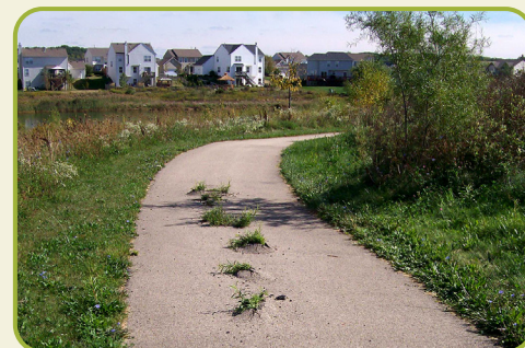
Tree root/shoot growth to be removed to prevent asphalt damage
