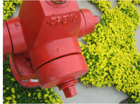
The Water/Sewer Utilities Operating Division maintains over 2,100 hydrants in the Village.
