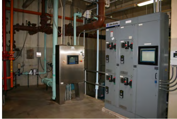
SCADA system at Wastewater Treatment Facility
