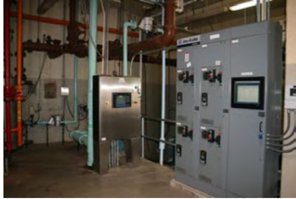
SCADA system at Wastewater Treatment Facility
