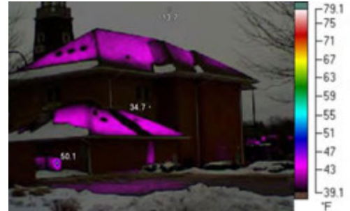
Thermal Image of Historic Village Hall identifying heat loss, provided by the Internal Services Division.
